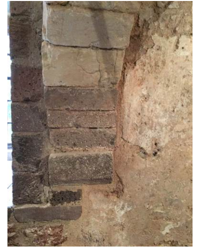
Twisted arch due the corbel being moved for later window reveal
