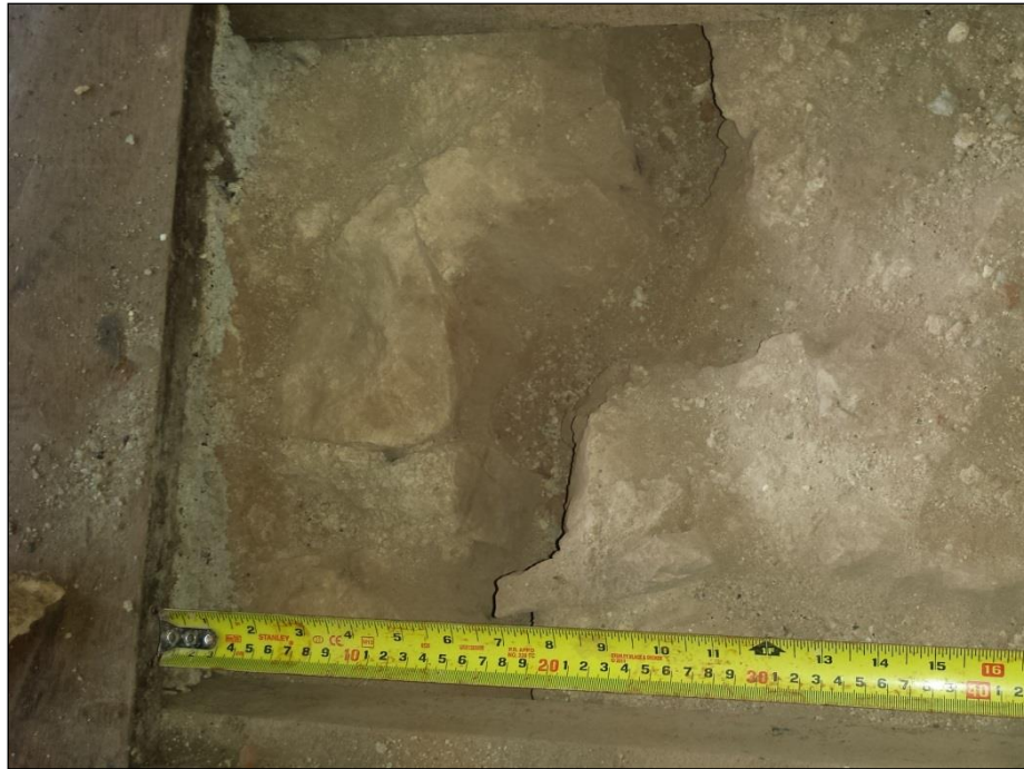
Image of the crack prior to cleaning out
