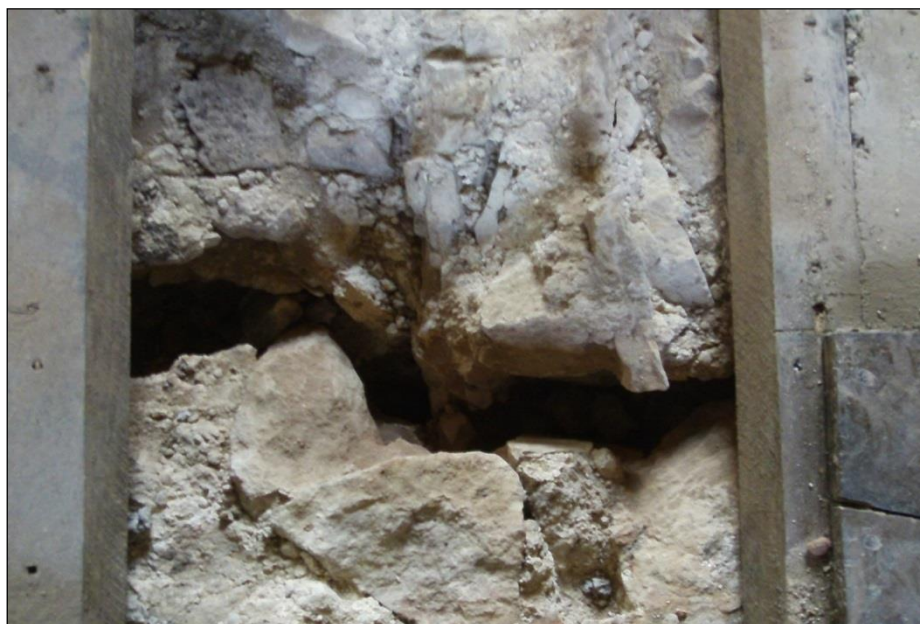
The trial pit and crack following vacuuming
