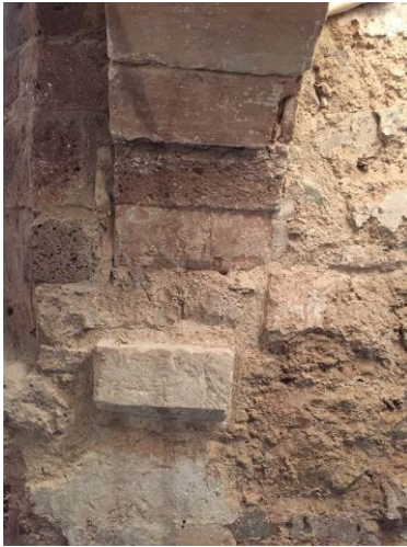
Misaligned arch with corbel
