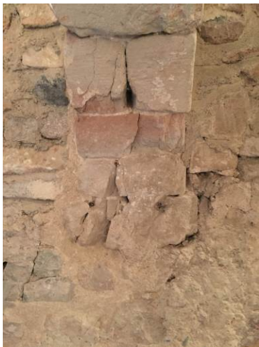
Fractured stones and corbel to rib.
