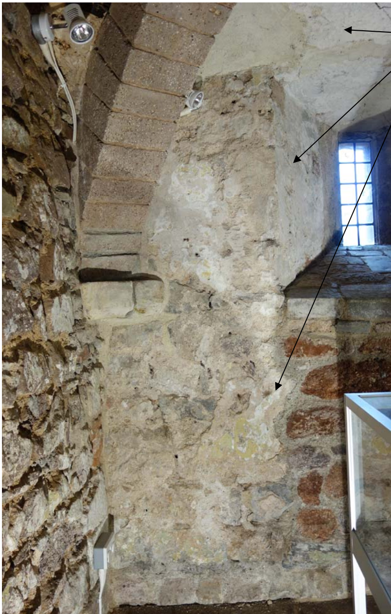
View of west wall showing original plaster on the ceiling and walls
