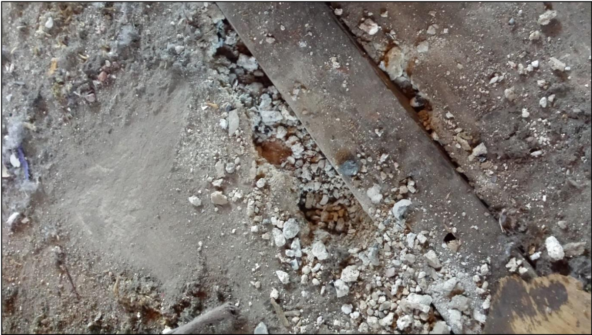
An image of the grey mix with small areas of the upper crust broken through.
