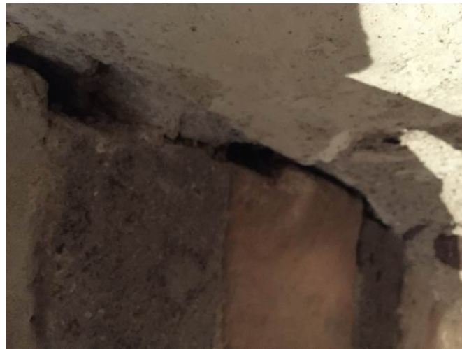
Ribs are not always tight to the vaulting.
